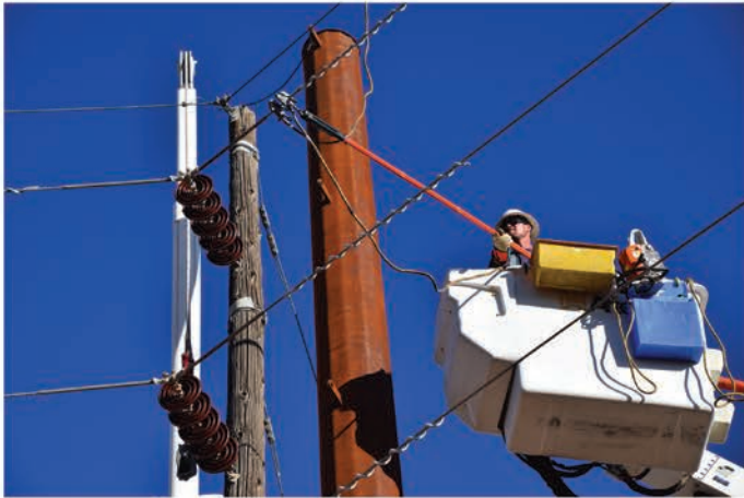
SSVEC lineworker Dylan Layton begins the process of moving a line during a pole replacement project in the San Simon area on December 20, 2018.
