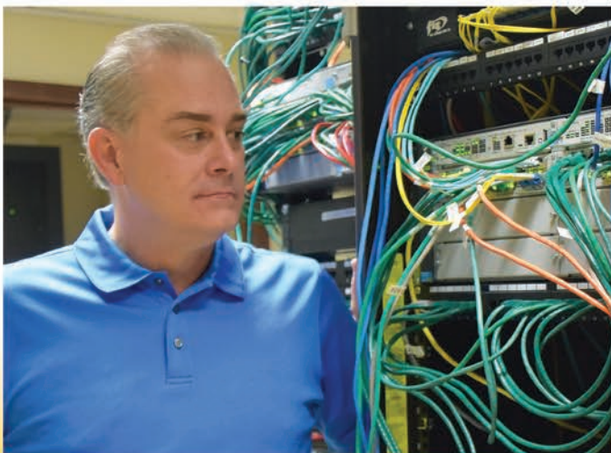
Orson Garnsey, Chief Information and Technology Officer, inspects servers in the Sierra Vista computer room.
