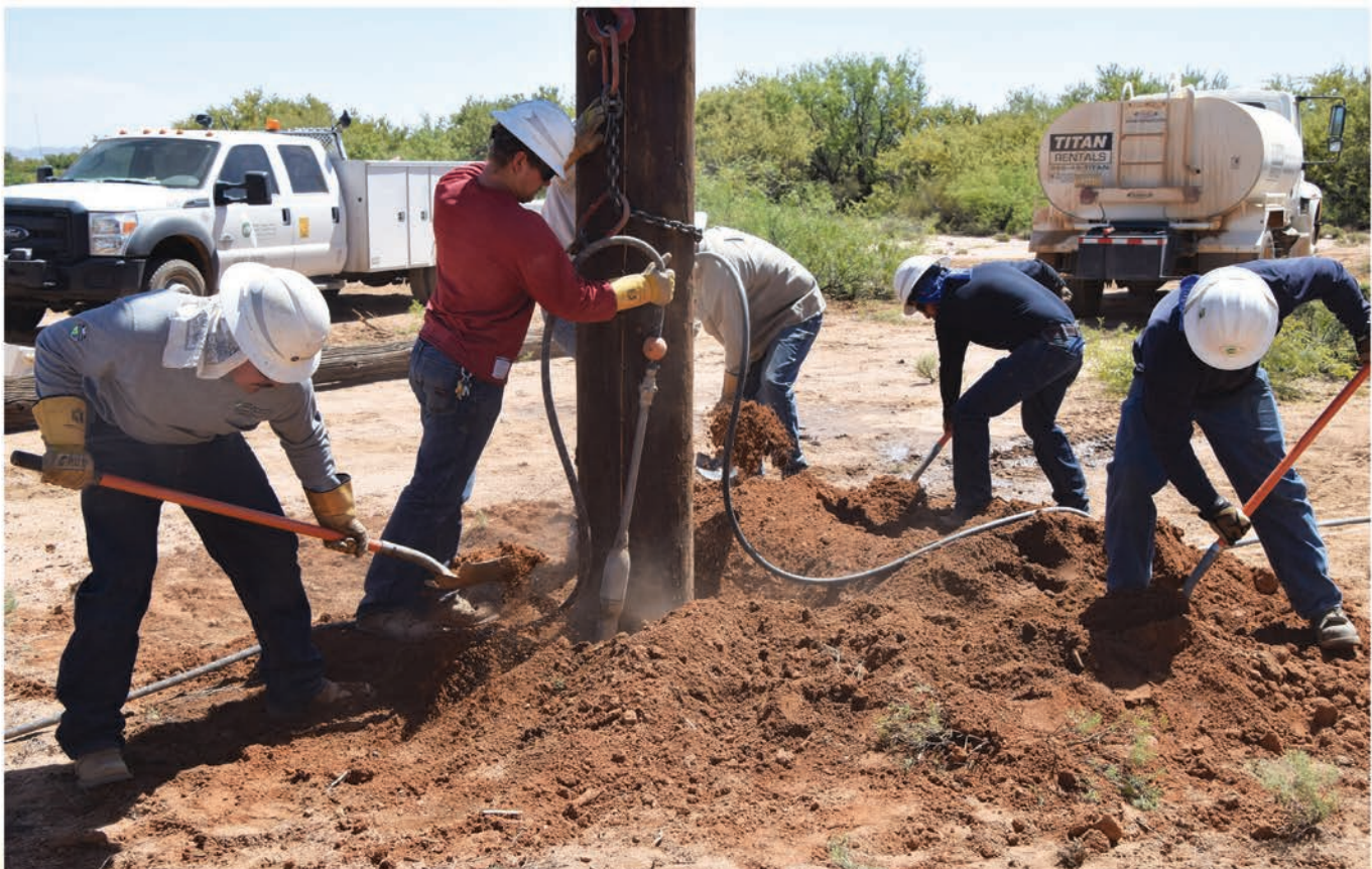
Once a new pole is set, it's all hands on deck as SSVEC linemen secure placement of a 65-foot pole as part of a pole replacement project outside of Bowie on May 21, 2018. Those tamping the pole include, from the left, Chuy Hernandez, Blake Rhodes, Clinton Welch, Luis Montano, and Emile Brunelle.
