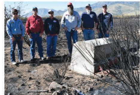
SSVEC lineworkers responded April 27, 2018 to a brush fire in Hereford. Multiple firefighting agencies responded to the scene. The Sulphur Springs crew headed into the fire field to take down a transformer before it fell off the pole and spilled oil. They also rerouted power lines from wooden poles which were either burning or were about to catch on fire. Members of SSVEC's crew include, from left, Tyler Rios, Nathan Hodges, David Clark, Zack Jouett, Eddie Soule, and Eric Jones.
