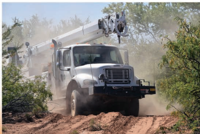
A SSVEC truck makes its way to a remote worksite during a pole replacement project in May, 2018.
